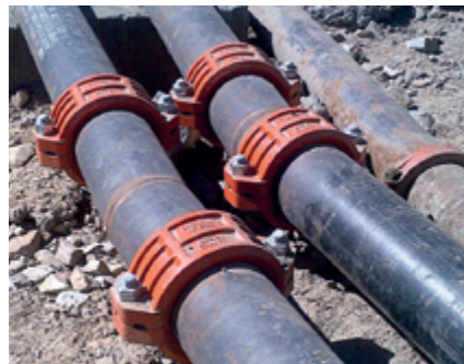
Model RX-3000 Couplings used in conjunction with Sch. 80 pipe line, Cerro Lindo Mine, Peru.
