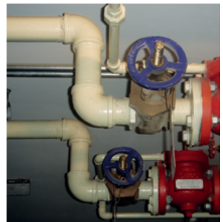
Fire Protection, 101 Building, Taipei, Taiwan
