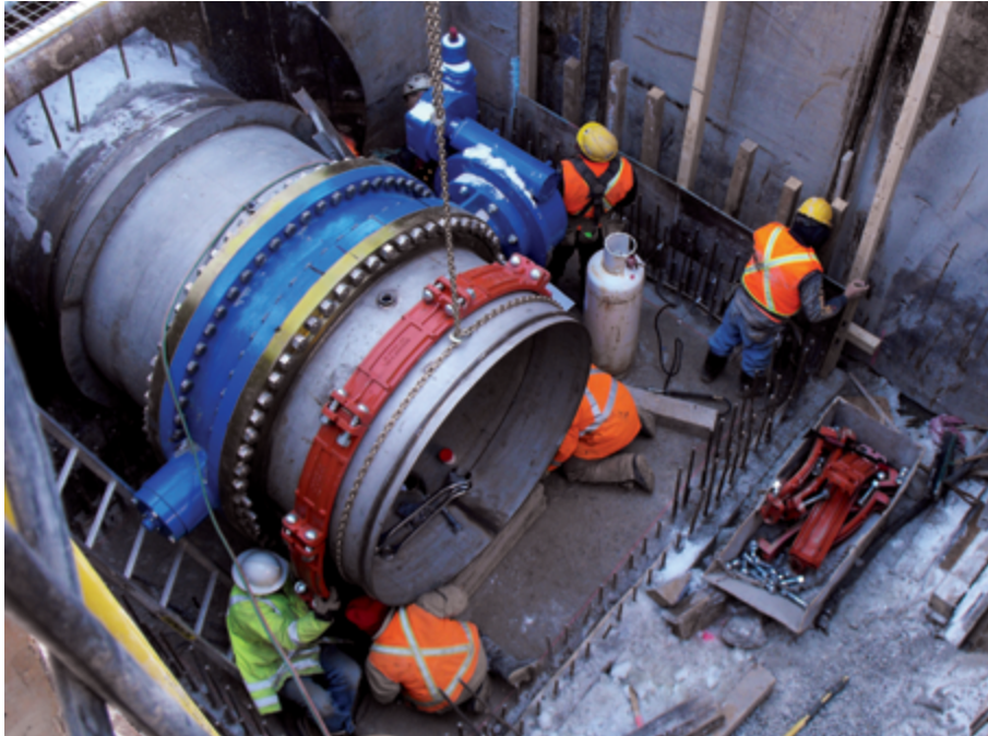
72" R-88 couplings used in F. J. Horgan Treatment Plant, Ontario Canada
