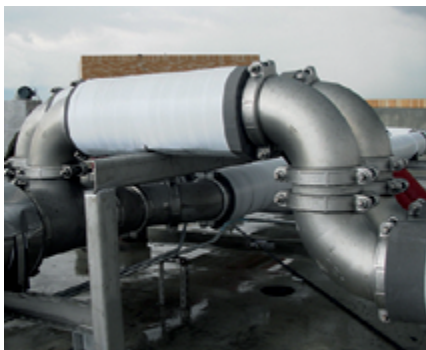
Water Supply, Chi Mei Medical Center, Liouying Branch, Tainan, Taiwan
