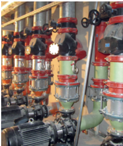
HVAC, IGS Building, Taipei, Taiwan
