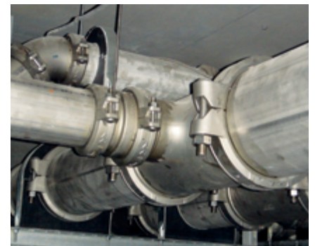
HVAC, Taichung City Government Office, Taichung, Taiwan
