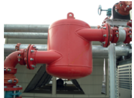
HVAC, Emergency Operations Center, Taipei, Taiwan
