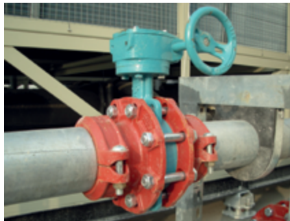
HVAC, Emergency Operations Center, Taipei, Taiwan
