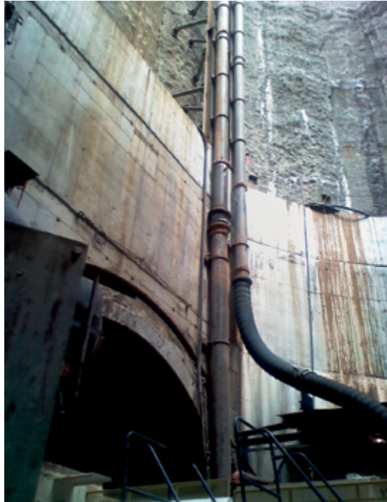
Shaft Piping, Portland East Side CSO Tunnel, USA
