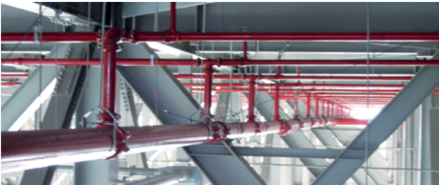
Fire Protection, Evergreen Aviation Hangar 2, Taoyuan, Taiwan
