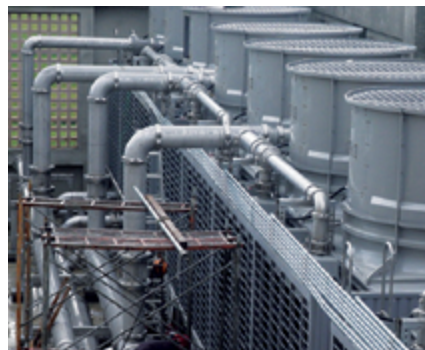
HVAC, Chi Mei Medical Center, Liouying Branch, Tainan, Taiwan
